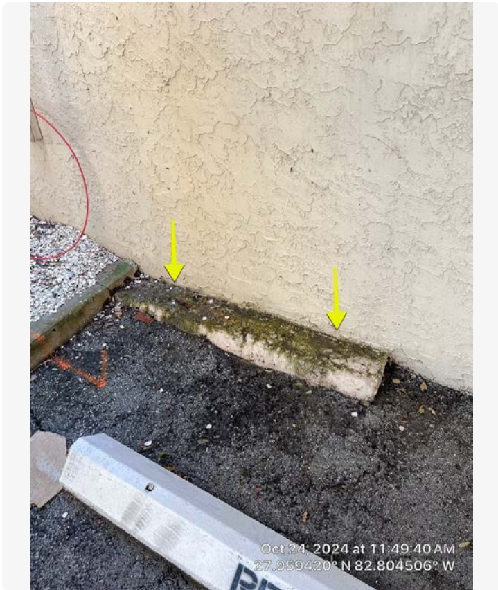
Northern corner of the west building elevation. Indications of water accumulation at base of building.
