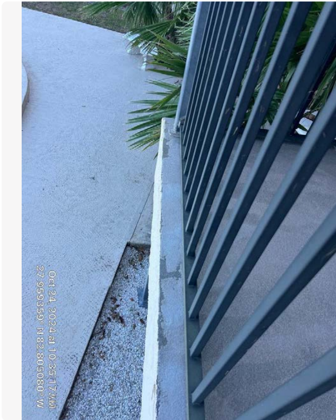
Deteriorating coatings observed on Unit 8 balcony slab edge.
