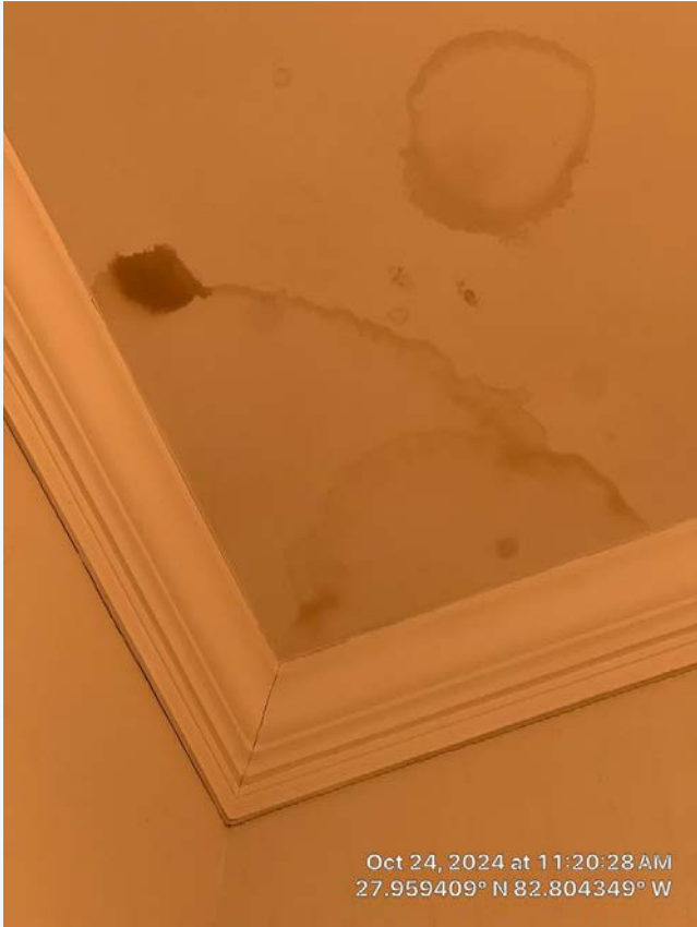
Water leak observed at 1st floor of Unit 4 interior.
