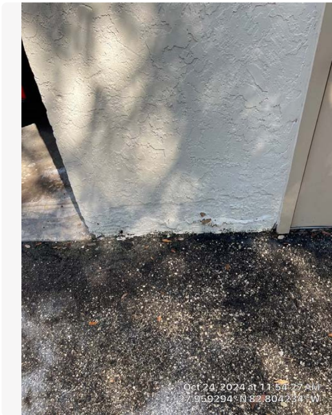
Garage unit 2. Water damage to stucco noted.
