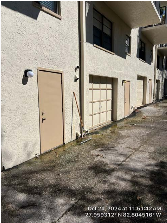
South elevation. Units 5 and 6 garage area. Water noted pooling.
