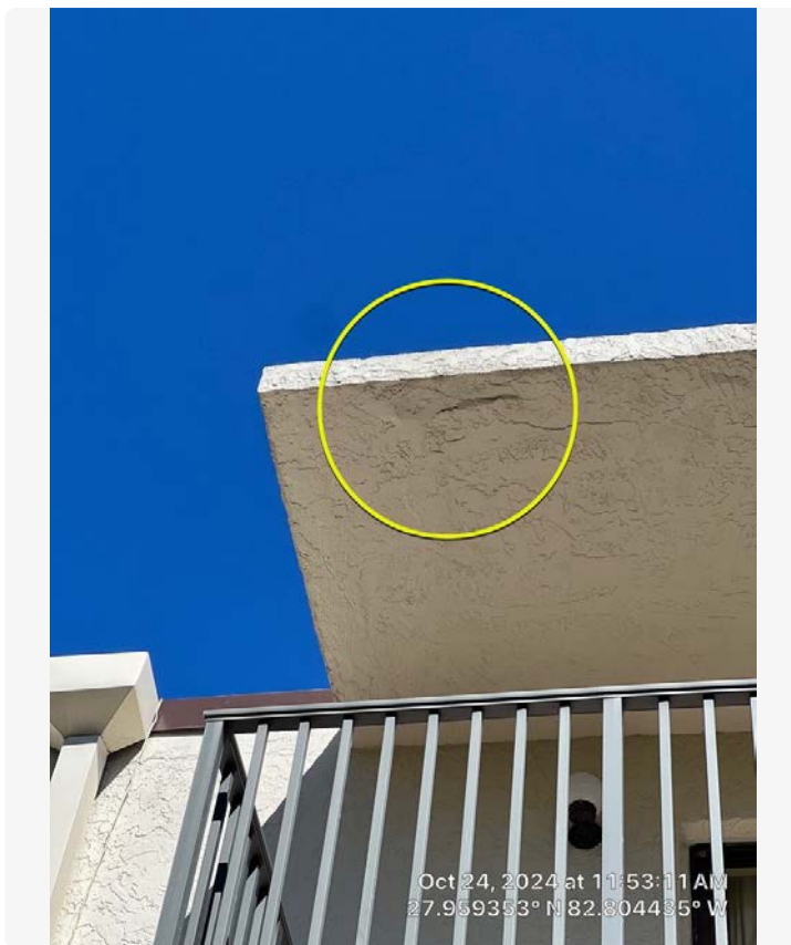
Unit 5 upper balcony roof. Possible water intrusion and stucco delamination. (South rear elevation)
