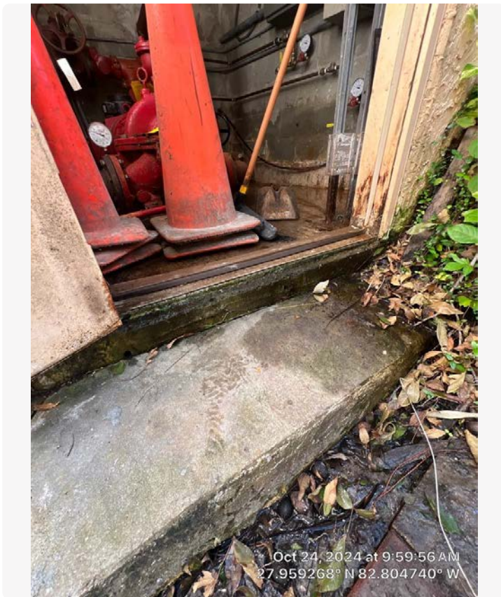
Pump room entrance. Water intrusion is obvious and the doorframe is showing signs of severe corrosion.
