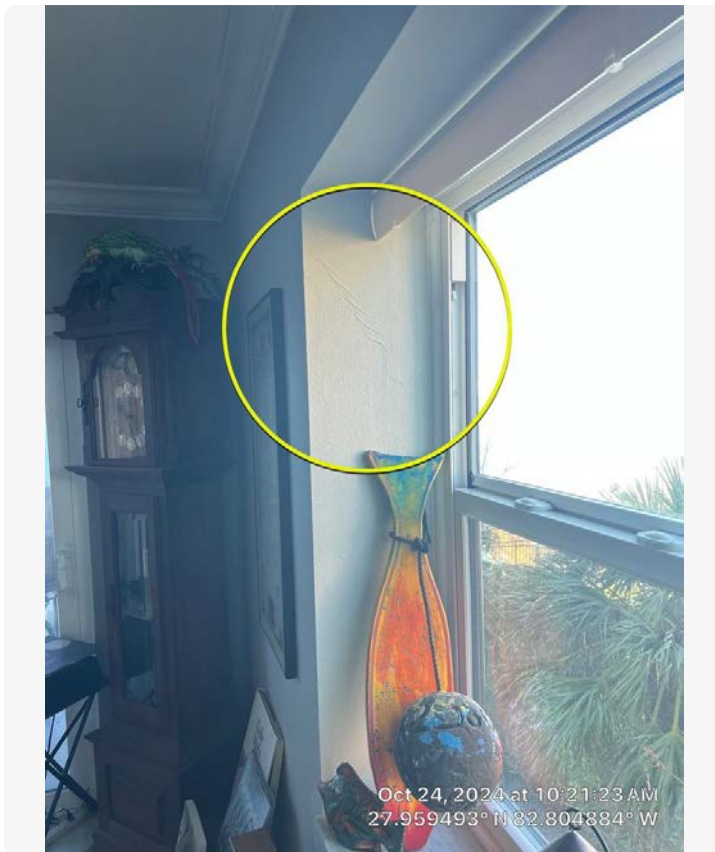
Water intrusion damage on north window in Unit 9.
