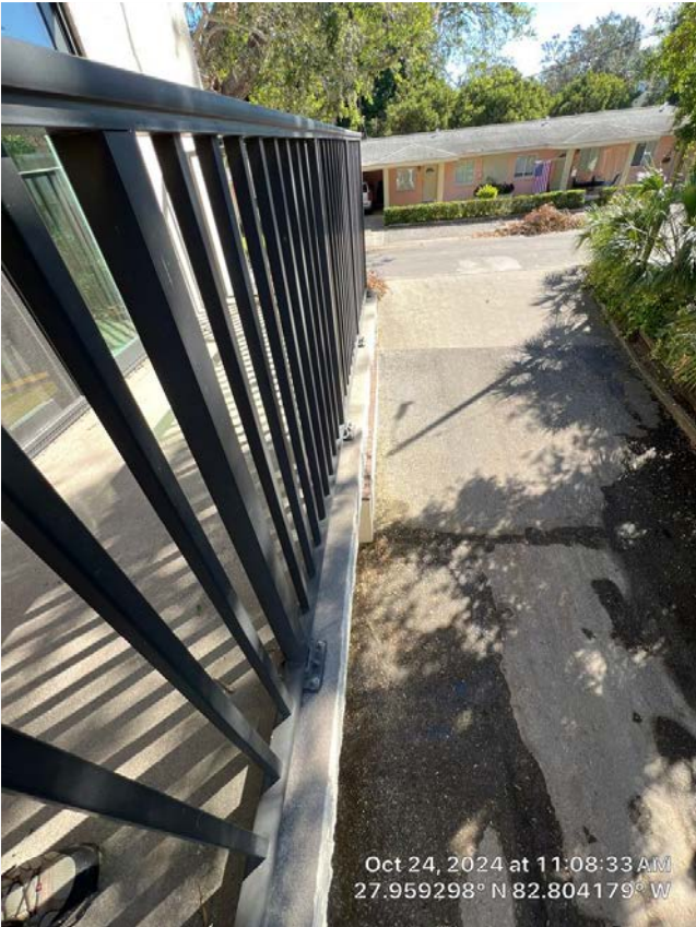
Unit 1 balcony slab edge.
