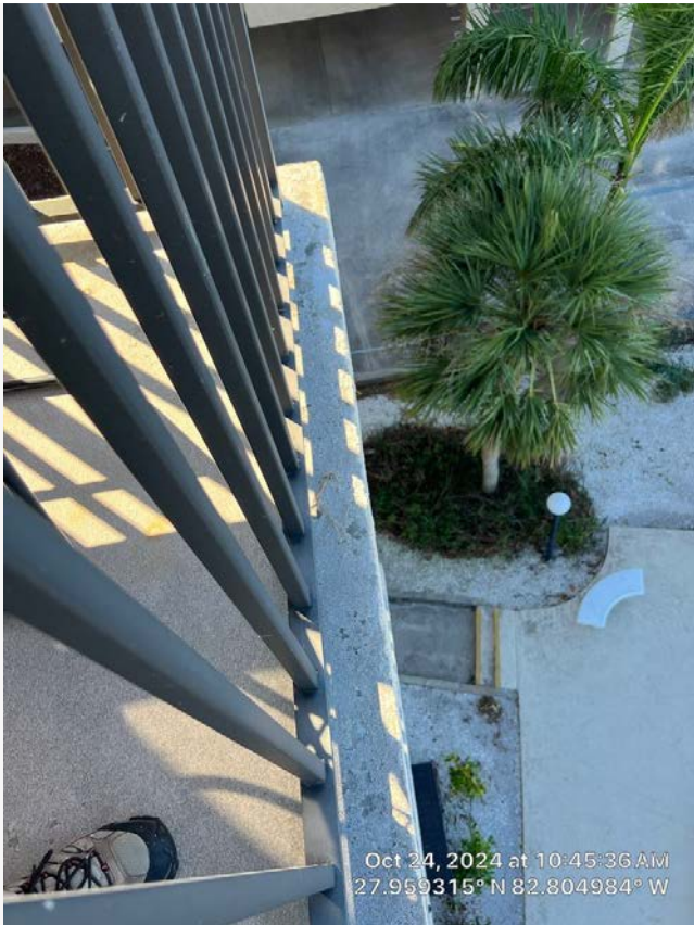
Deteriorating coatings observed on balcony slab edge Unit 14.
