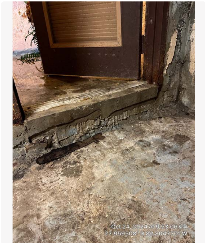
Elevator room door surround. Long-term water intrusion is evident at this location.
