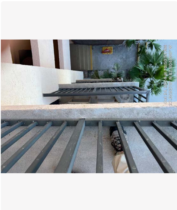
Close-up of coating of balcony Unit 13.
