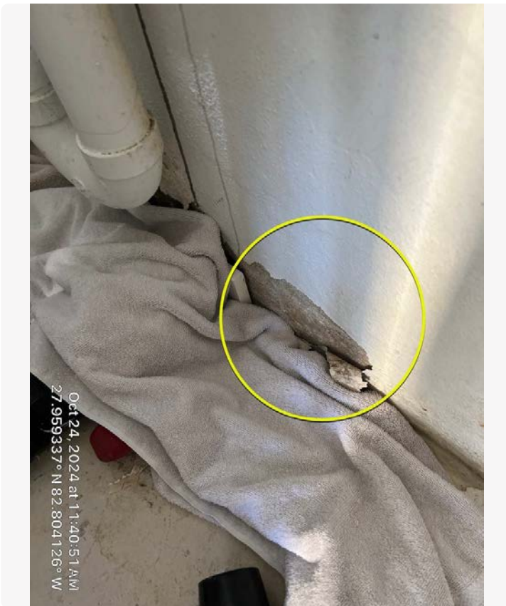
Unit 1 garage. Small leak. Owner estimates a gallon per hour during storm.
