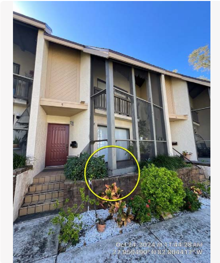
Unit 5 porch enclosure. Damage to wooden posts observed at this location.
