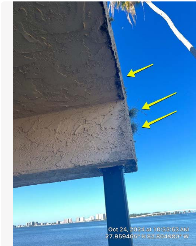
Unit 7 balcony roof. Moisture and plant life observed at this location.
