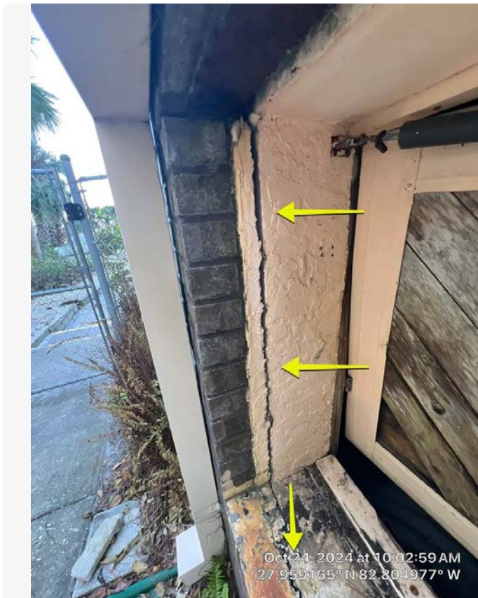
South elevation crawl space door. A large crack was observed between the building facade and the underlying concrete. This should be repaired to prevent additional water intrusion and degradation of the facade.
