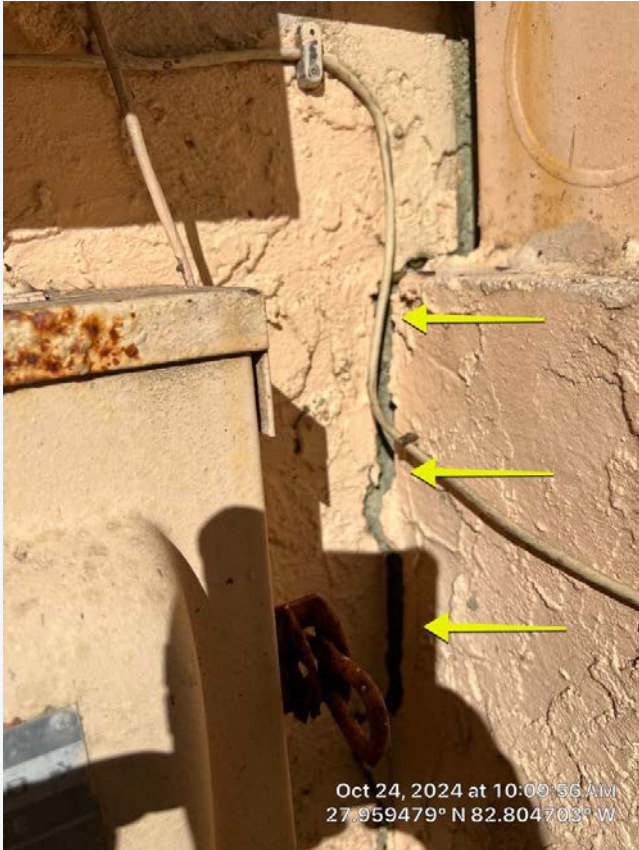
Front east elevation. Cracking in concrete observed.
