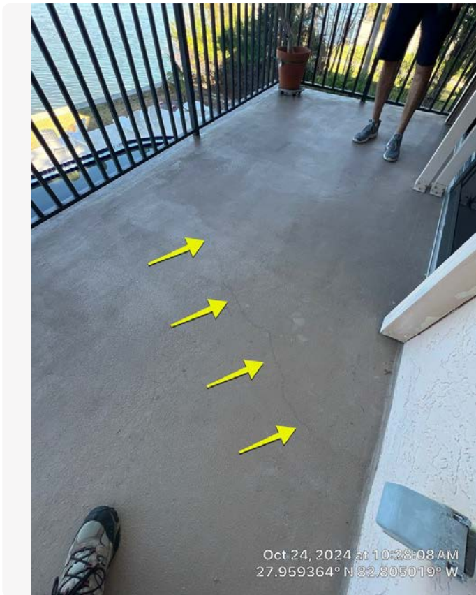
Minor crack observed on balcony for Unit 10. This is not a structural issue and no action is required, however the deck should be coated with a waterproof membrane which will bridge this crack and prevent water intrusion into the slab.
