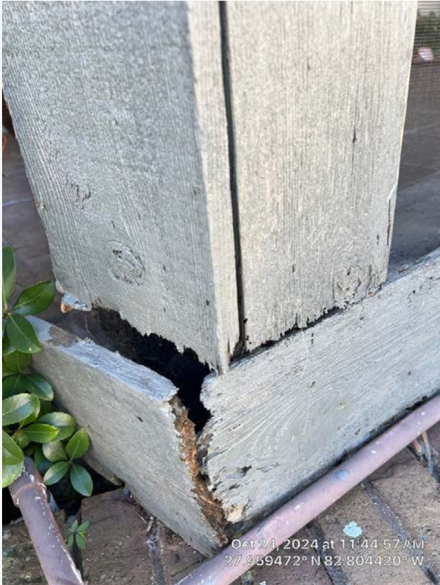
Unit 5 porch enclosure. Damage to wooden posts observed at this location.
