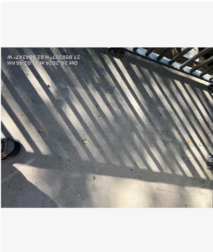
Unit 2 south balcony, Typical conditions observed throughout the building.
