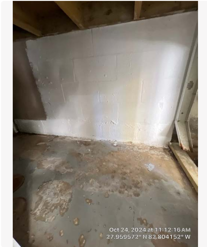
Water intrusion location through walls in garage of unit 3.
