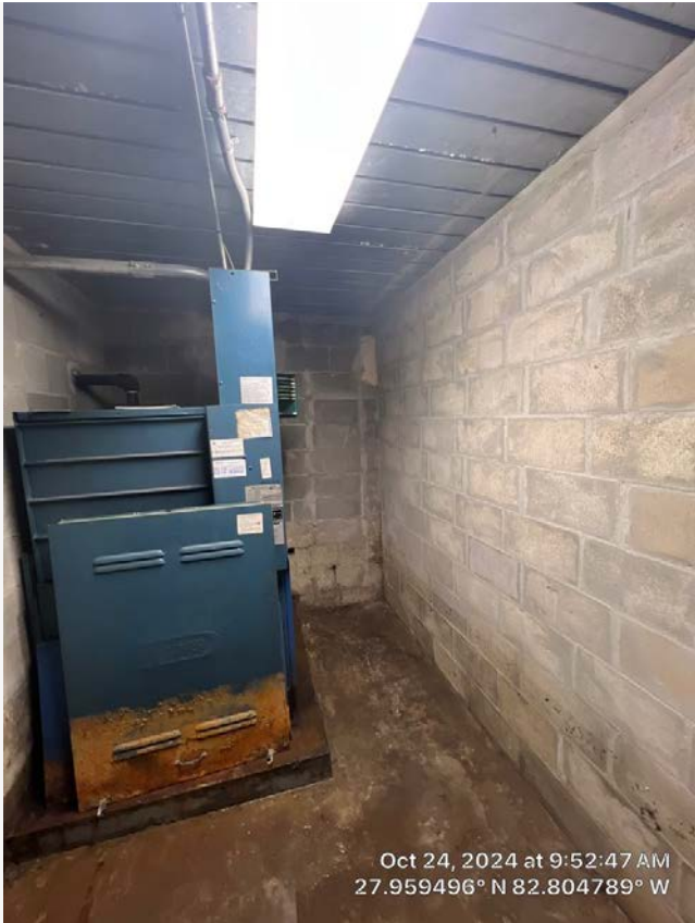
Elevator room. There is standing water in this location .
