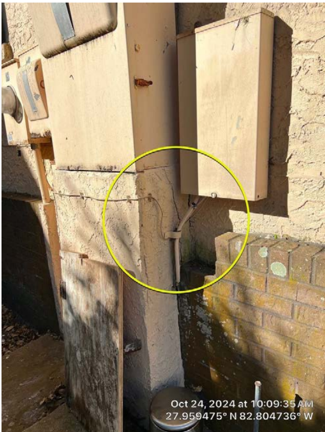
Front east elevation. Cracking in stucco observed. This crack should be repaired to prevent moisture-induced deterioration of the stucco.
