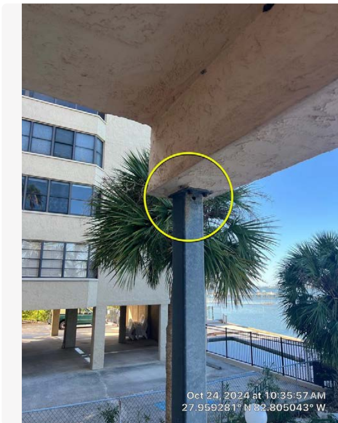
Minor corrosion observed on metal support column. Balcony of Unit 8. Right now this is minor surface rusting, however the steel needs to be repainted to help prevent further corrosion induced deterioration of the post.
