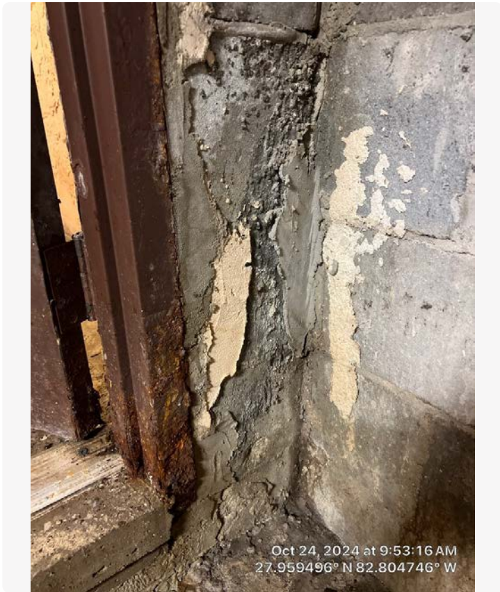
Corrosion and concrete damage noted at the door surround location in the elevator room. Long-term water intrusion is evident at this location.
