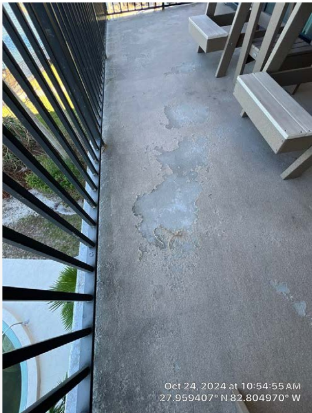
Waterproofing has reached the end of its serviceable life.
