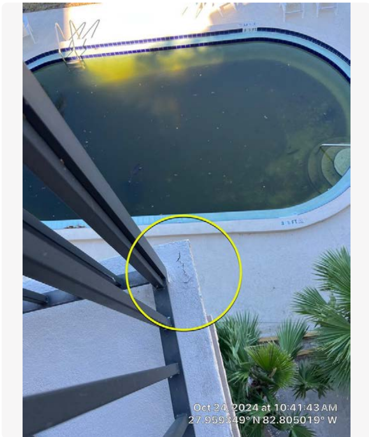
Minor cracks observed on the southwestern corner of balcony Unit 12. The coatings on the deck appear to generally be in good condition, however this slab edge should be touched up to prevent water intrusion.
