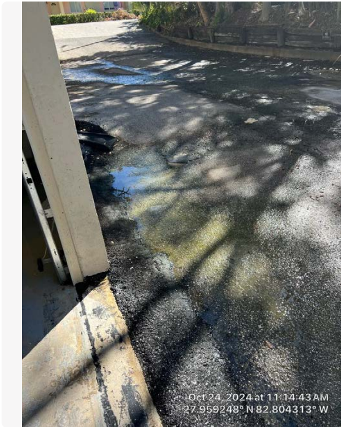
Outside of Unit 3. This water is reported to be from some unknown source other than rain. The source is unknown.
