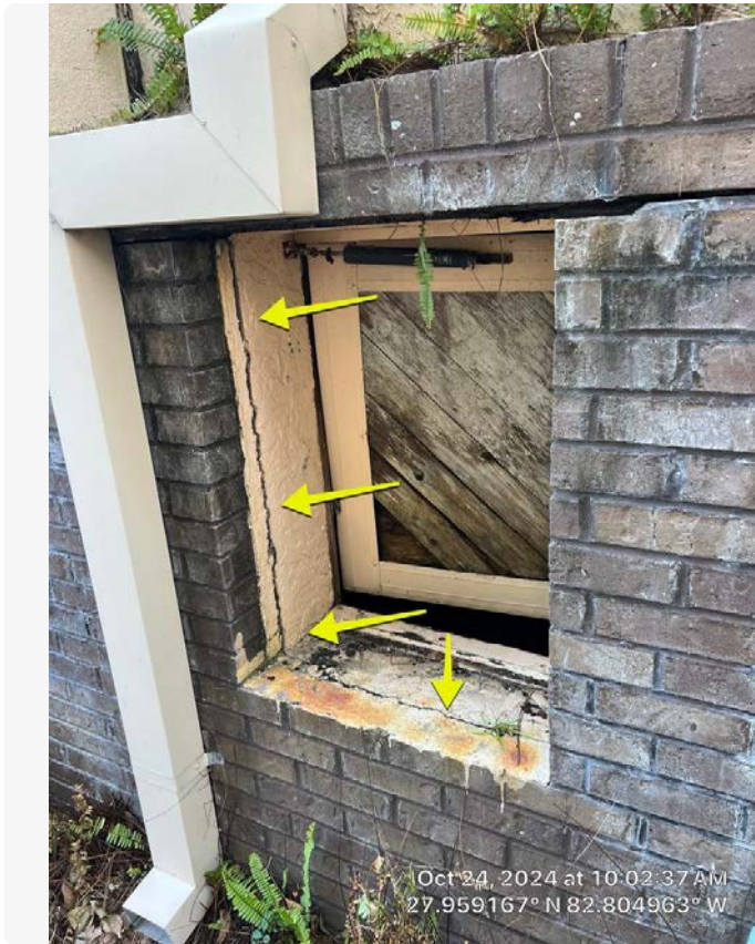
South elevation crawl space door. A large crack was observed between the building facade and the underlying concrete. This should be repaired to prevent additional water intrusion and degradation of the facade.
